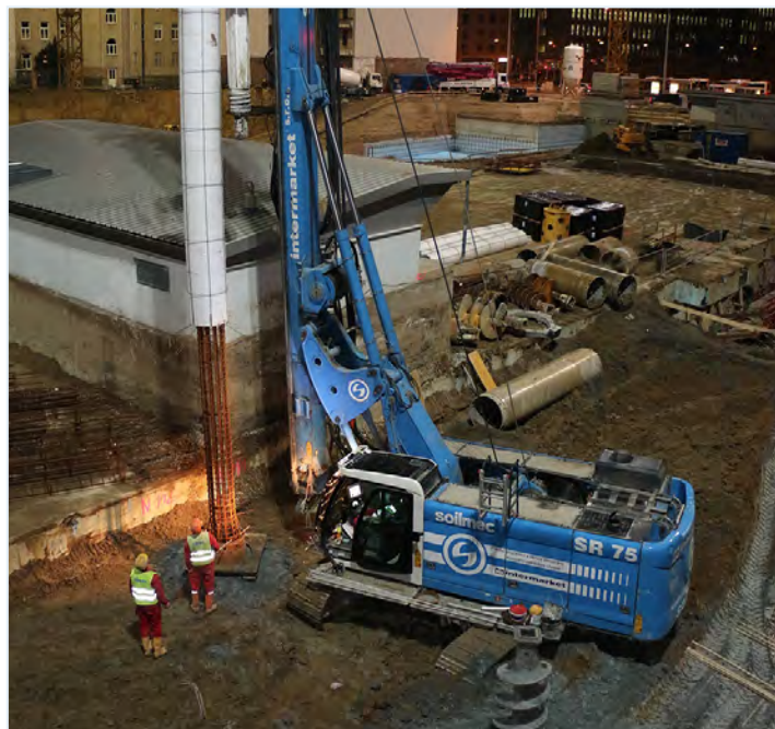
Soilmec SR-75 drilling rig equipped with DMS in action in the very center of Vienna for the "Trienna" project - Austria
