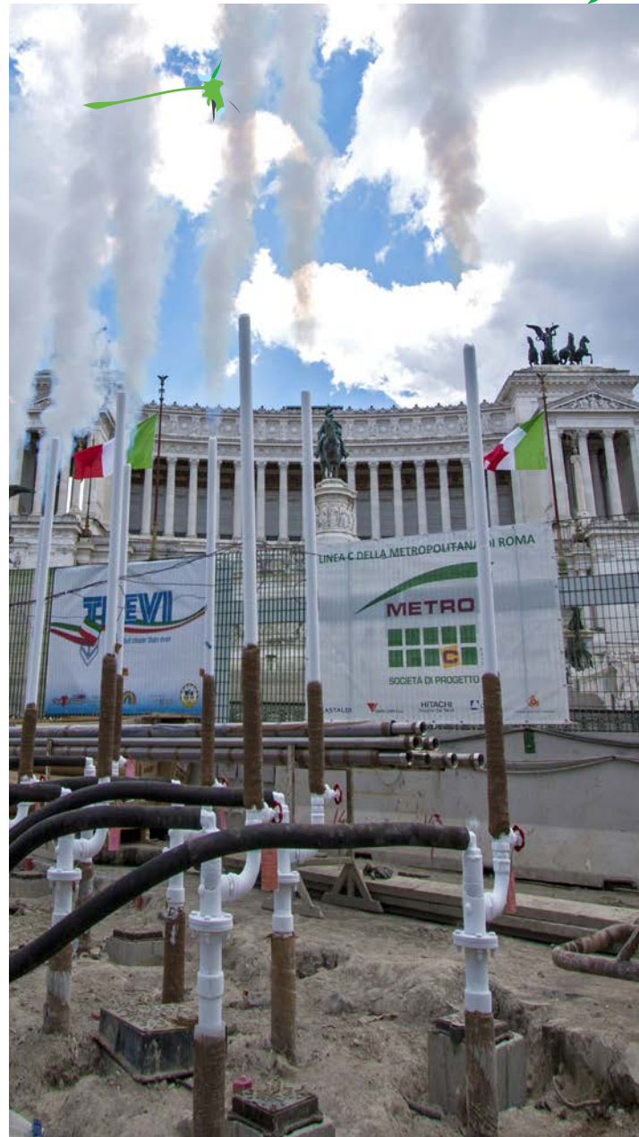
Freezing technology for the new station of Piazza Venezia, Rome metro, C Line _ Italy
