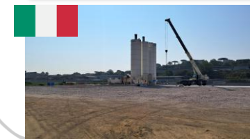
Perimetral containment of the Malagrotta landfill (Rome)
